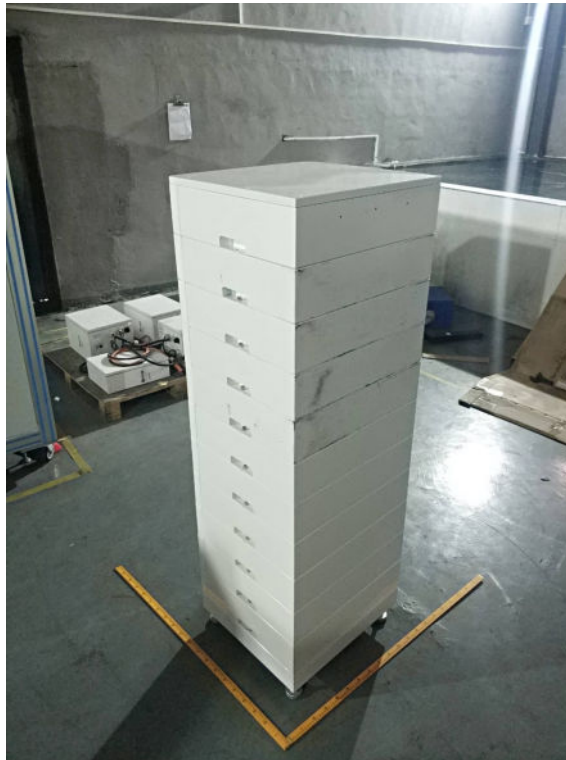
General view-2 of battery
